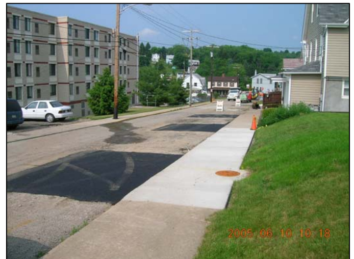
View of the manhole cover of the Early Warning System in the repaired sidewalk. (June 10, 2005)
