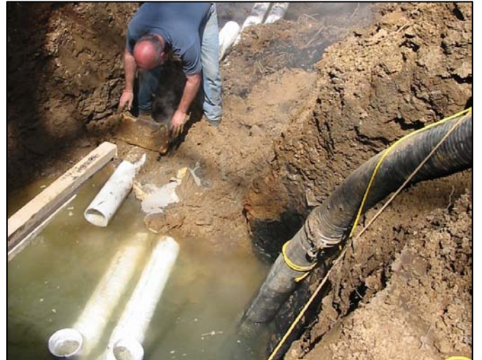
A temporary gravity drain was installed at Test Pit 1 before installation of the permanent Primary Drain. (April 10, 2005)
