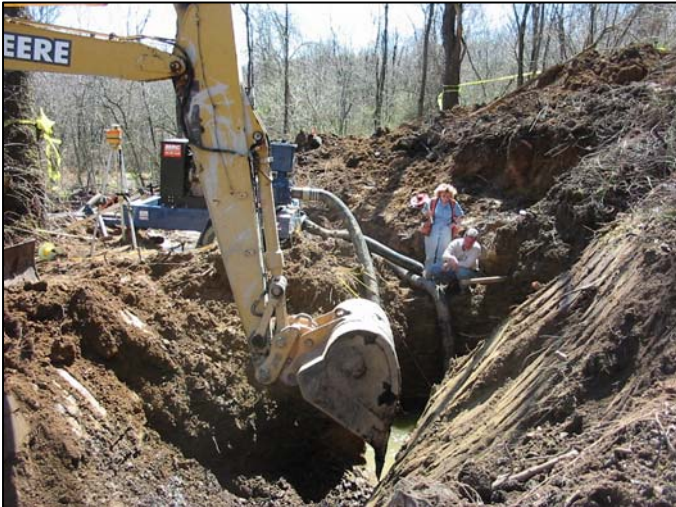
Test pits excavated with pumping conducted to determine favorable locations for Primary and Secondary Drains. (April 8, 2005)
