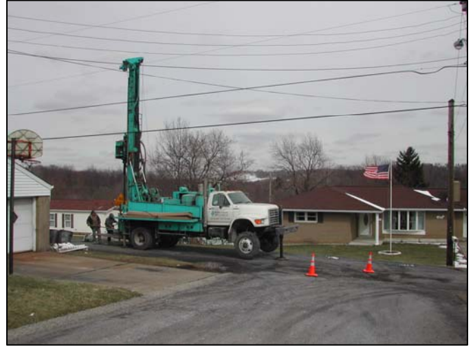
Piezometers installed as part of hydrogeologic investigation. (March 10, 2005 – photo by Rich Beam, BAMR)
