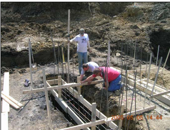
Placing the form and rebar for the Primary Drain concrete footers at Test Pit 1. (May 5, 2005)
