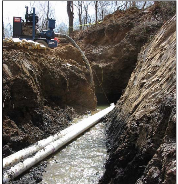
Pipes placed in Test Pit 1 to temporarily drain the mine water by gravity. (April 10, 2005)
