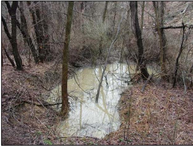
Subsidence depression receiving drainage from "Miller Run" prior to Test Pit 3 excavation. (March 3, 2005)
