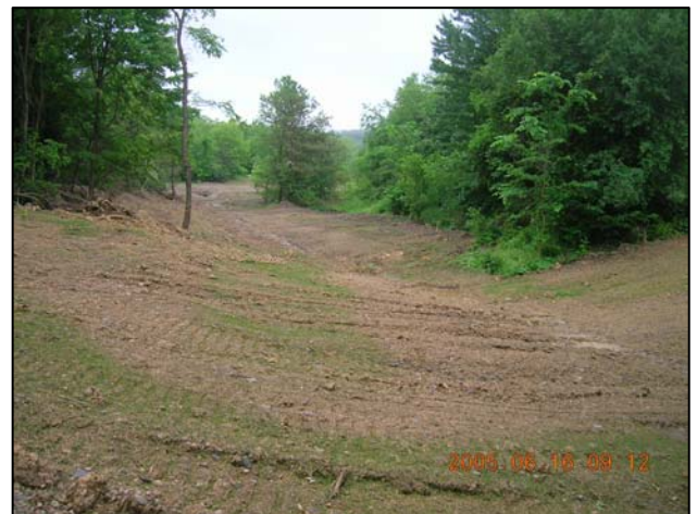
View from Secondary Drain manhole looking down channel towards access road/"Miller Run". (June 16, 2005)
