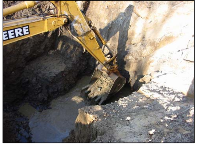
Excavating sump at Test Pit 3 for installation of Secondary Drain riser. (April 13, 2005)
